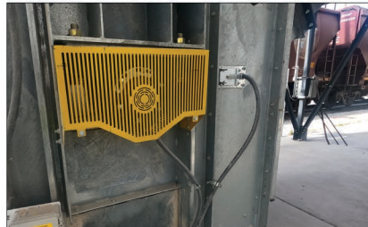
A couple of numerous bearing and rub block sensors in the hazard monitoring system.
