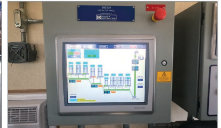
A touchscreen panel in the control room allows for easy monitoring and control.
