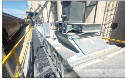
The system controls bin percentage gates to allow for accurate blending.
