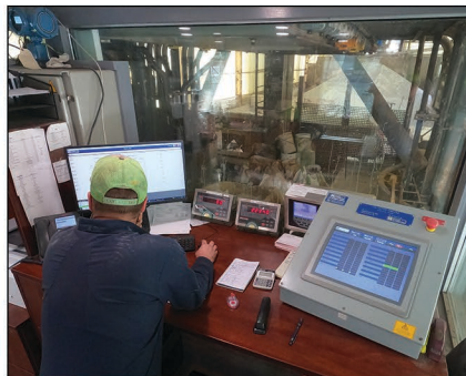
Control room with sloped 15" touchscreen and Plant Supervisor PSX software allows staff to accurately fulfill product dispensing orders.
