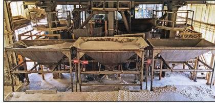
Three dry product hoppers on scales that feed the two liquid blenders.
