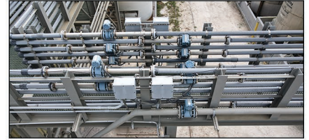
A few of the mag meters located in different areas used to measure various products.
