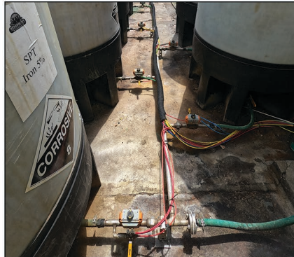
Plumbing and valves for the micro ingredients.
