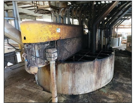
One of two blenders to manufacture product from dry and liquid additives.
